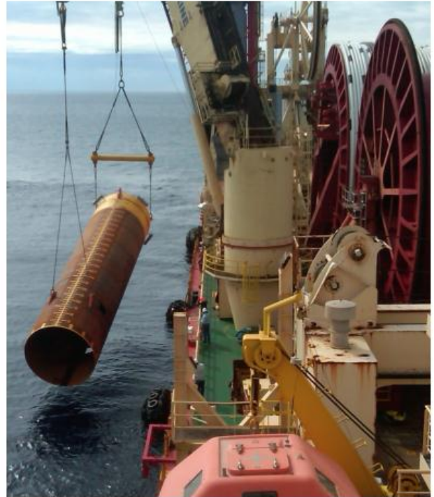
Express installing suction piles in the Walker Ridge block of the Gulf of Mexico
