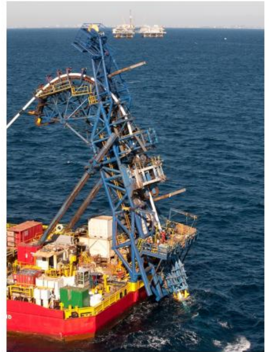
Intrepid performed pipelay and diving operations off the California coast during the fourth quarter.
