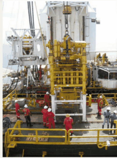
Q4000 Intervention Riser System in operation
