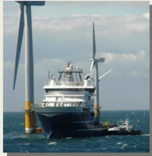
Deep Cygnus performing trenching and cable burial operations at the Greater Gabbard Offshore Wind Farm in the North Sea
