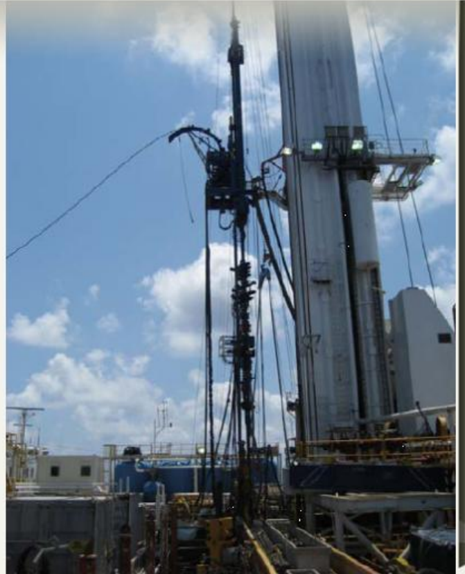
Coiled tubing operations for Marubeni on a deepwater well in the Gulf of Mexico
