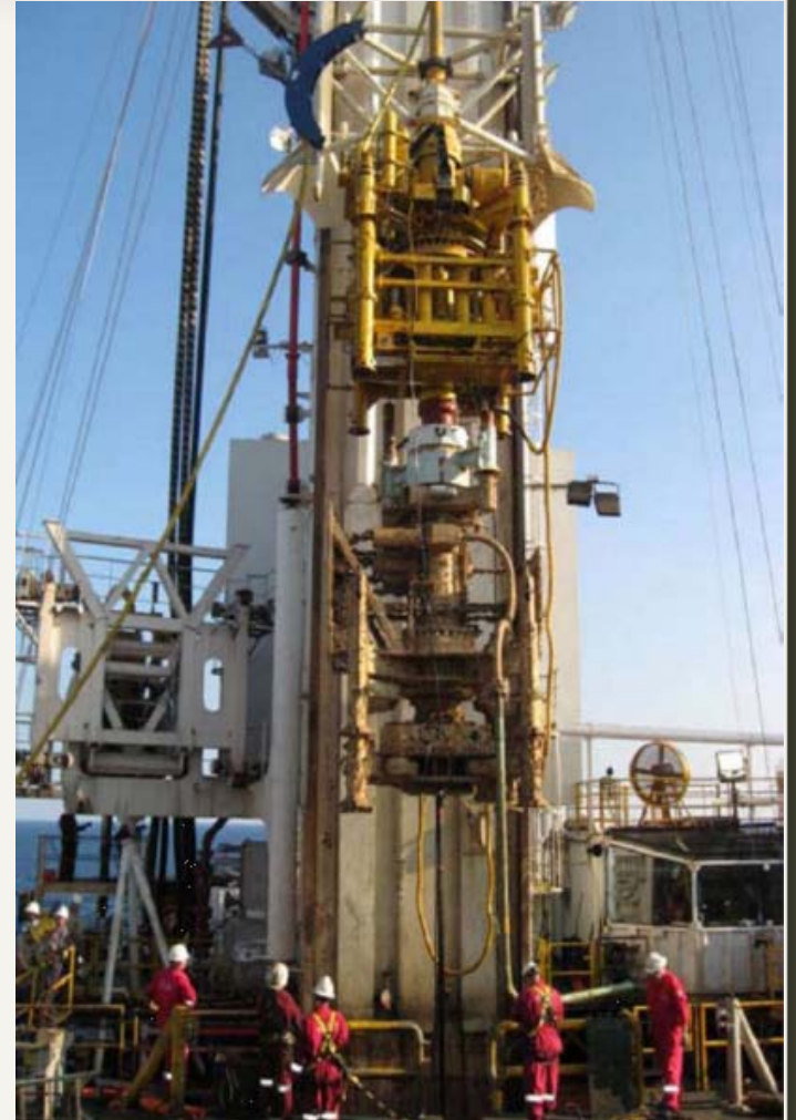
Well Ops' Intervention Riser System recovers a tubing head spool with tubing in one recovery trip
