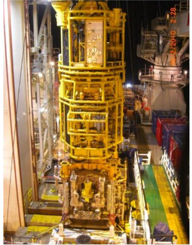
Wellhead, tree and SIL lower intervention package recovered by the MPT on the Well Enhancer
