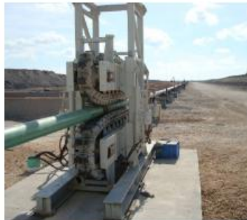
Automated pipe tension system
