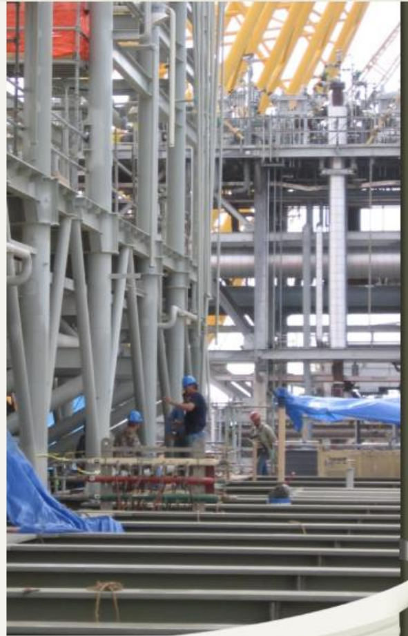
HPI pipe racks connecting production modules to buoy system
