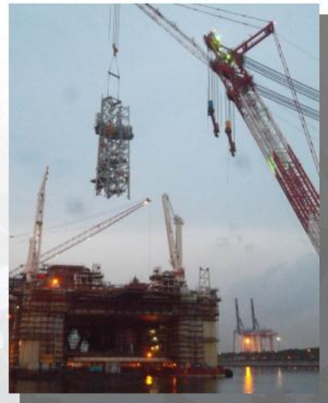
NOV tower being installed on the Q5000
