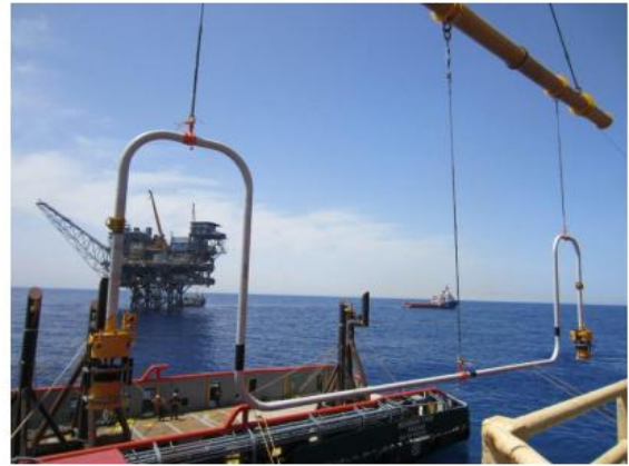
Express installing a jumper in Noble Energy's Noa field off the Israel coast.
