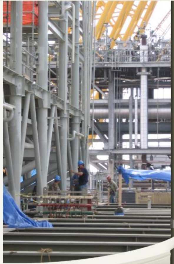
HPI pipe racks connecting production modules to buoy system
