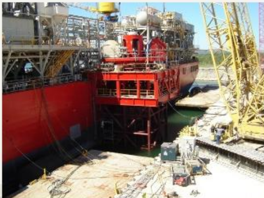
Disconnectable Transfer System
