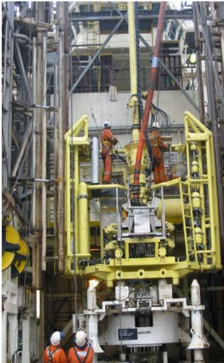
5 1/8" SIL in the Seawell Derrick
