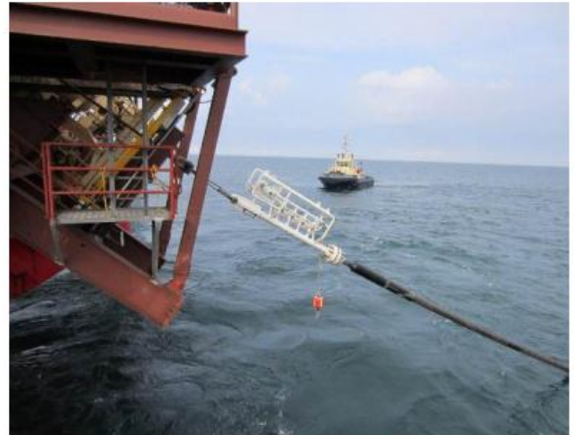
Express lowering a pipeline pullhead as part of a North Sea installation operation.
