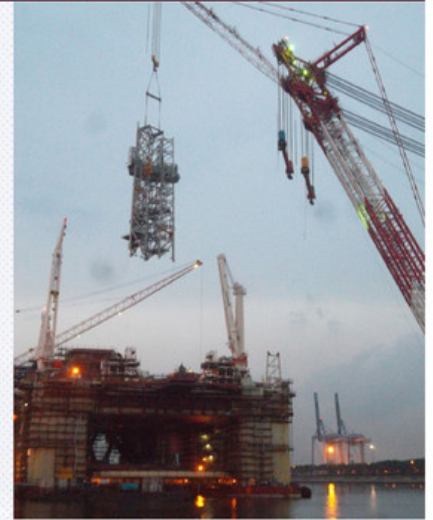
NOV tower being installed on the Q5000
