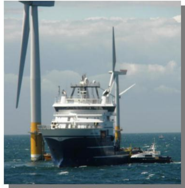
Deep Cygnus performing trenching and cable burial operations at the Greater Gabbard Offshore Wind Farm in the North Sea
