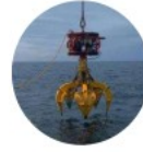
IROV Boulder Grabs Remotely operated robotic grabs specially developed to relocate seabed boulders to prepare an Offshore Wind Farm site for construction
